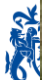
Work carried out to form the car park to Ford Cottage looking east
